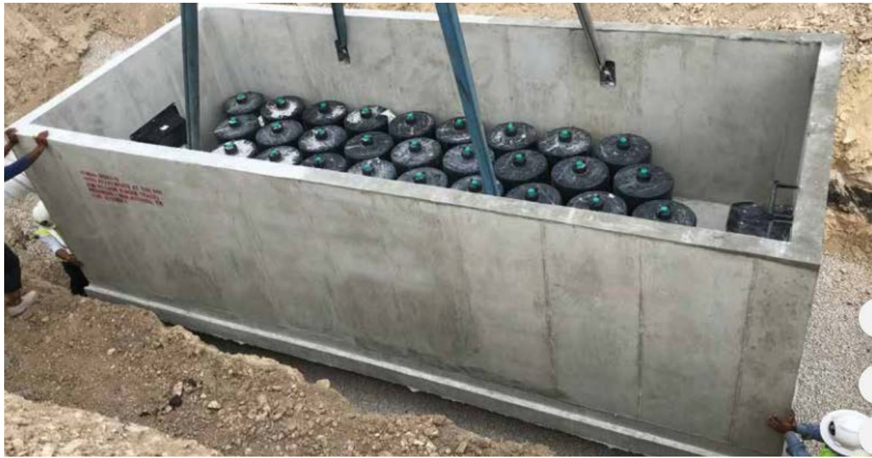
Figure 5. Example of a Filtration System in the Field.
