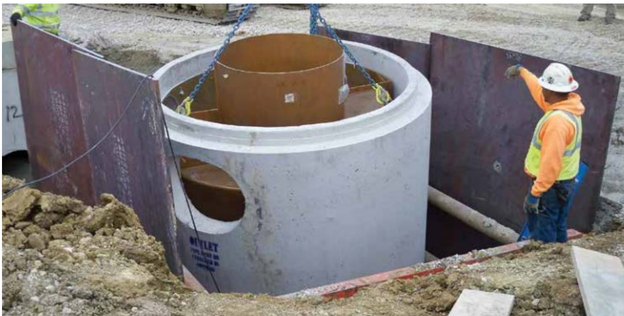
Figure 3. Example of a Hydrodynamic Separation Device (HDS) in the Field.
